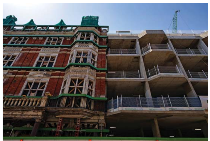
ABOVE: Marring up of the listed façade to 90–93 Piccadilly and the new reinforced concrete frame, enabling the removal of the façade and staircase retention system.
