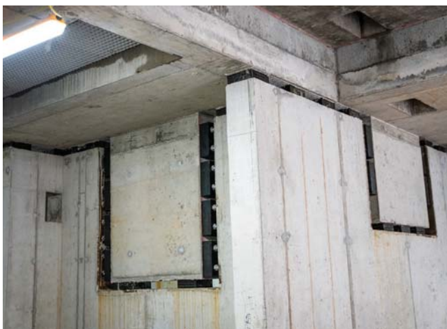
ABOVE: Cambridge House acoustic pads providing further vibration attenuation and separation within the reinforced concrete core for Building 3.
